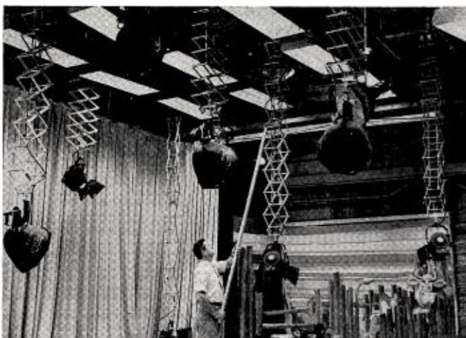
NEW "skyhook" lights, which can be regulated to any height, are one of WCAU-TV Philadelphia's Studio A lighting features. Station engineers report lights satisfactory under all conditions. The incandescent lights are attached to overhead power rails and may be suspended or angulated in any direction and can be moved to any direction on power rails with a minimum of effort. One man can set studio lighting in a minute or two. WCAU-TV is using a bank of 12 of these "skyhooks" along with several banks of overhead fluorescent lights, floor fluorescent floods and regular floor flood lights to give its studio daylight results.
